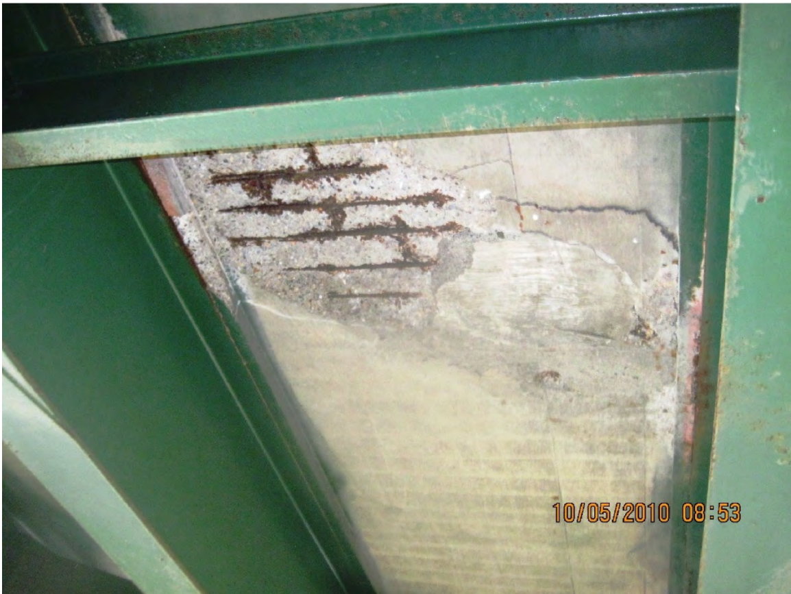
Localized Deck Deterioration
