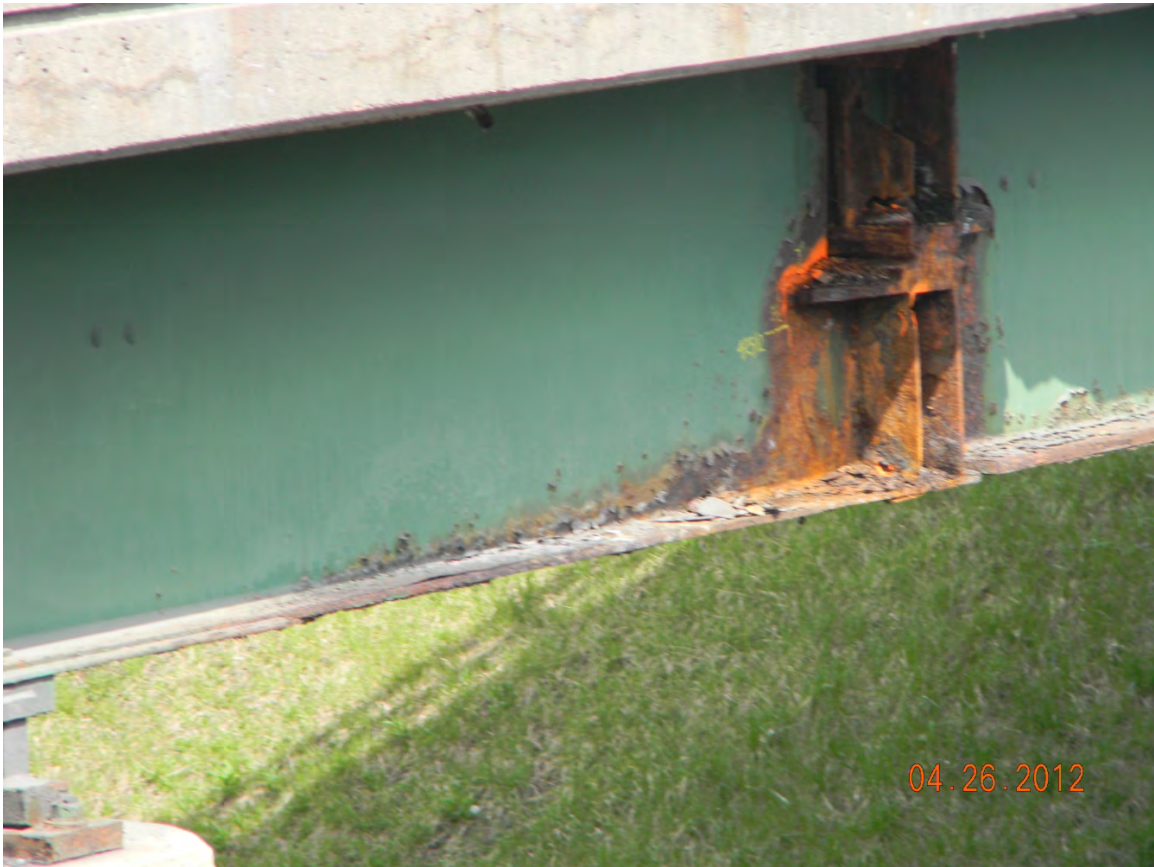
Cracking around Beam Support
